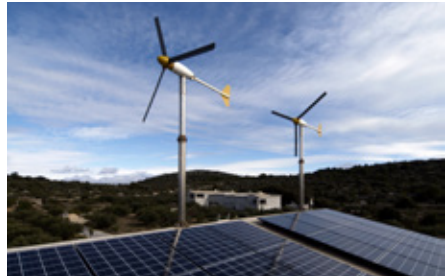
Solar Wind Hybrid Plant. Credit: Nenad Kajić used under CC BY-SA 4.0
