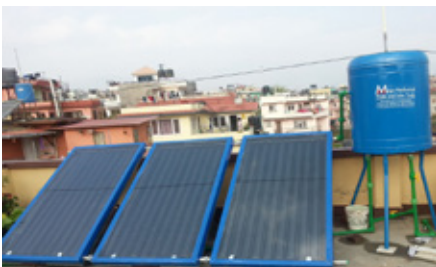
Solar Water Heating
