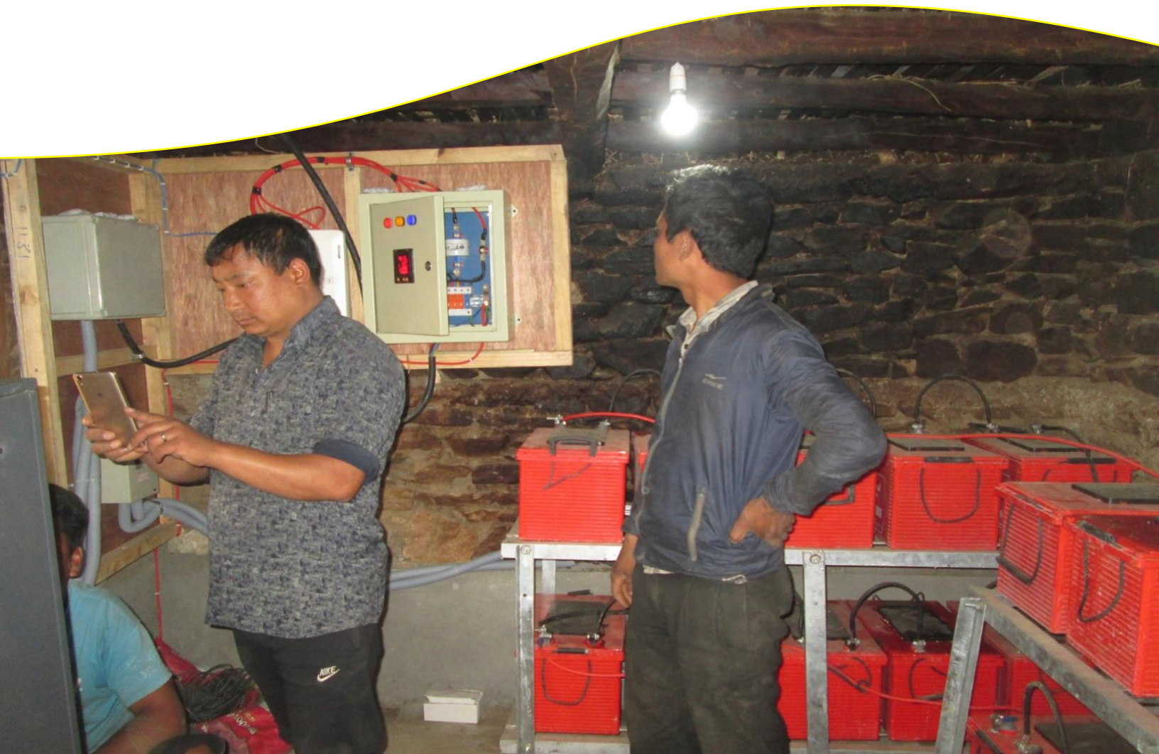
Power Testing of Installed Solar Mini Grid at Khanikhola, Kavre
