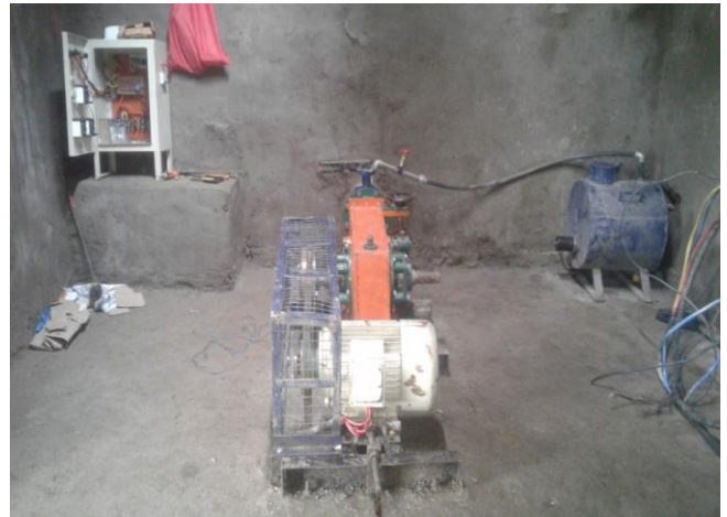
Installed Turbines and related accessories
