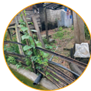
Grey water reclamation
