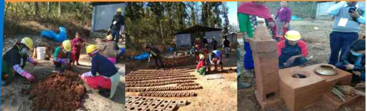
Participants Practicing the Construction of Different Types of ICS During the Practical Sessions
