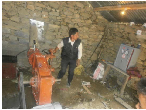
Figure 3 Powerhouse of IWM Electrification Project
